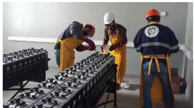
Monitoring the assets of the substation - battery inspection.
