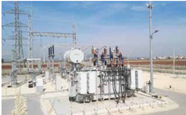
During the technical team's work at Al-Jalameh substation.
